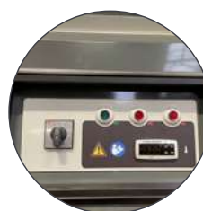
Panel de control
